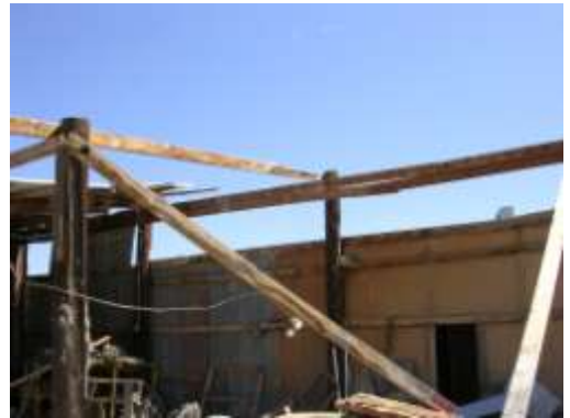
Barn damage from microburst in Pleasant Valley, NV area
