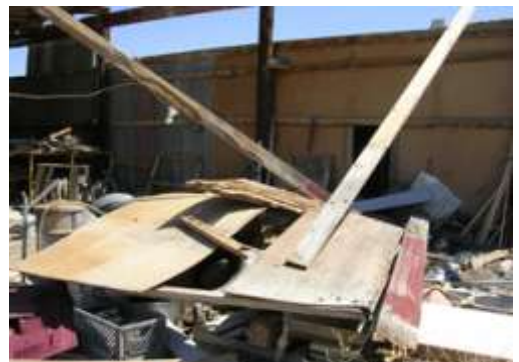
Barn damage from microburst in Pleasant Valley, NV area
